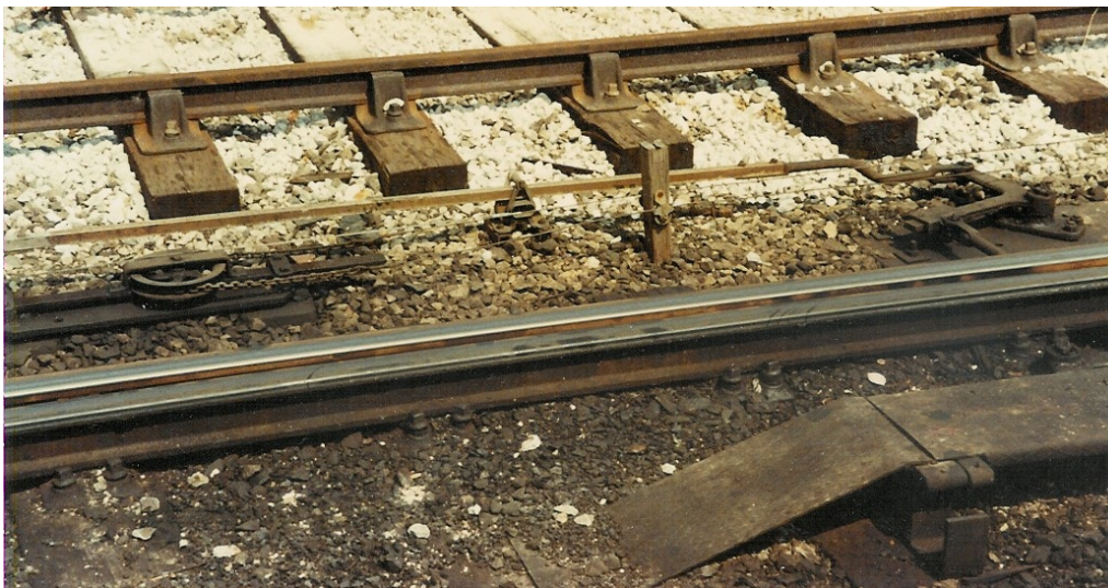
Figure 16B. Details on point rodding (channel section), an adjustable crank and signal wire pulley. The pulley is arranged to operate one of two ground signals, determined by the detectors (in Figure 16C) and "floats".
